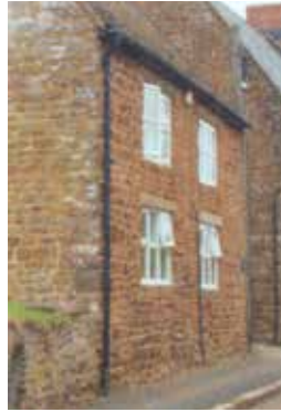
Black painted cast iron rainwater goods on rise and fall stirrup brackets
